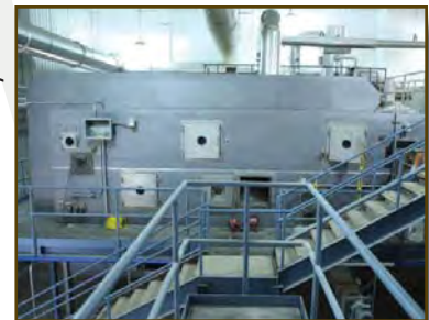
Biosolids Belt Dryer
