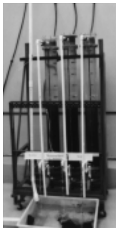
Technology utilized by Bolton & Menk may make compliance with new federal standards more affordable for cities.
