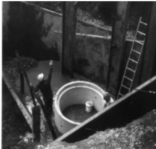
Jackson East River Interceptor Lift Station, 1995
