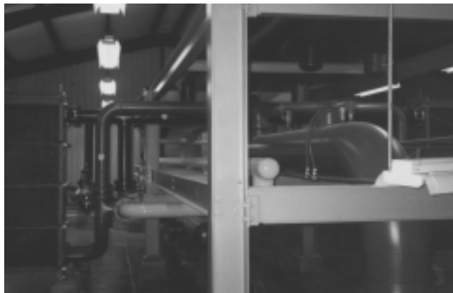
Waste heat facility shown with one of the heat exchange units and a portion of the interior piping system
