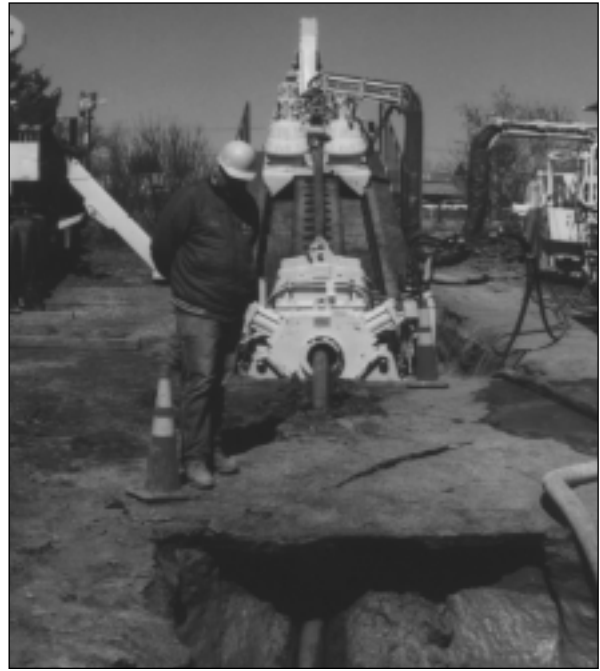
A Michaels Pipeline employee monitors the horizontal directional drilling unit used in the Saint Peter project.
