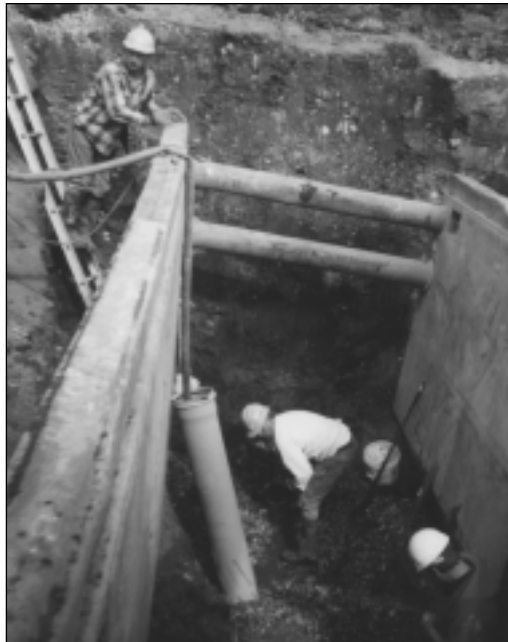
In Dundas, construction workers prepare to install sanitary sewer below the ground water table.
