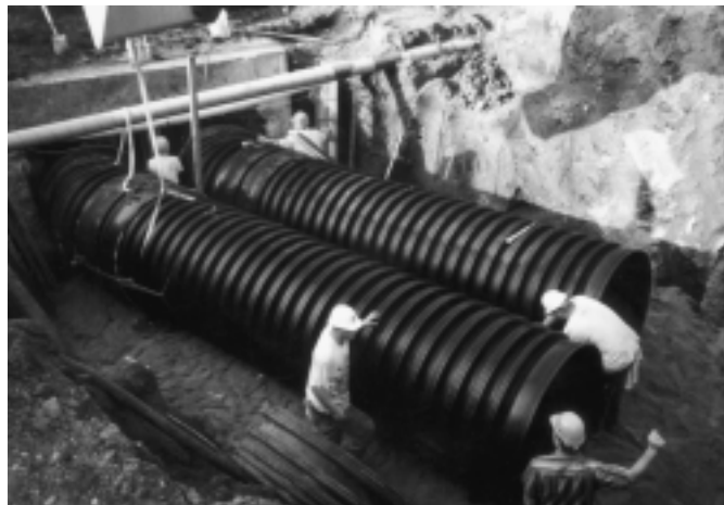
Placement of the dual pipe system on top of the 'aggregate pillow.'
