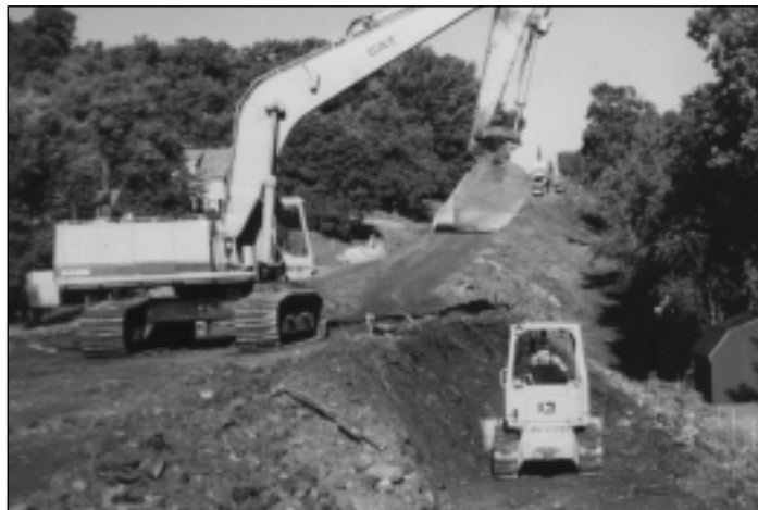
Grading of Dakota County Road 42 moves the the project toward a close.
